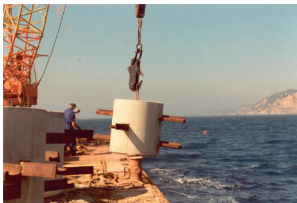
Fig. 3 Concrete reef modules with projecting steel beams such as railroad tracks are deployed in protected marine areas of Spain to discourage illegal trawling, so as to promote restoration of seagrass habitats and fish populations. Photograph Courtesy of Juan Goutayer.
